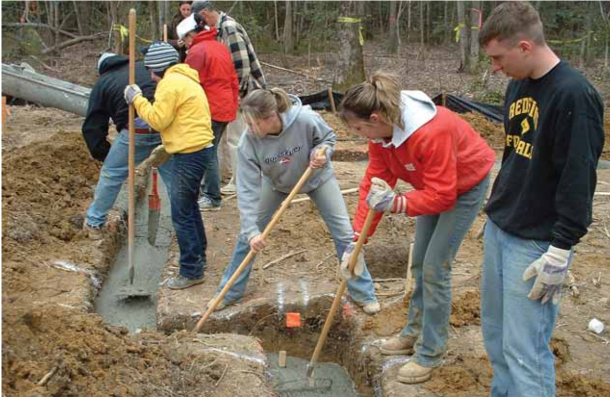
UNIVERSITY STUDENTS WORK ON THE FOUNDATION OF A HABITAT FOR HUMANITY HOME IN VIRGINIA
